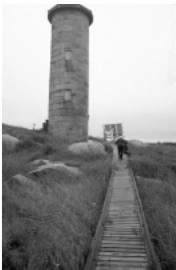
U.S. Fish and Wildlife Service rebuilds the boathouse, landing slip, walkway and historic light structure.
